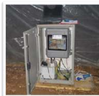
Data acquisition system
