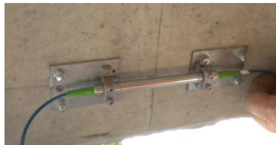
Fiber optic sensor mounted on bridge deck
