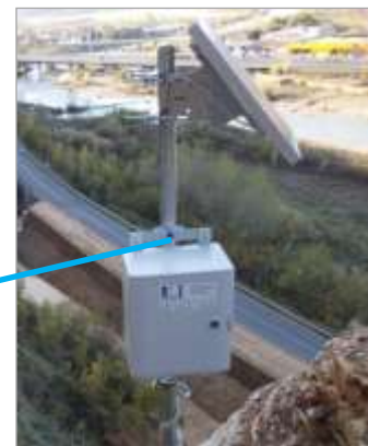
Warning station with GSM/GPRS modem connected to the maintenance department.
